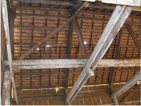
Holes in roof
